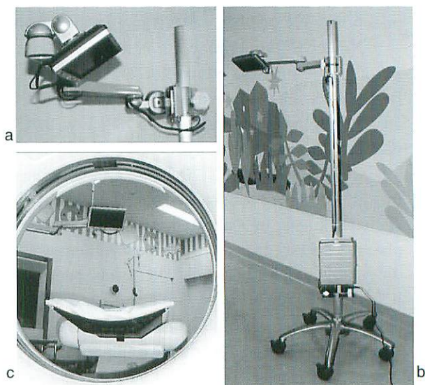
Fig.2 TV monitor system in CT unit of NCCHD
